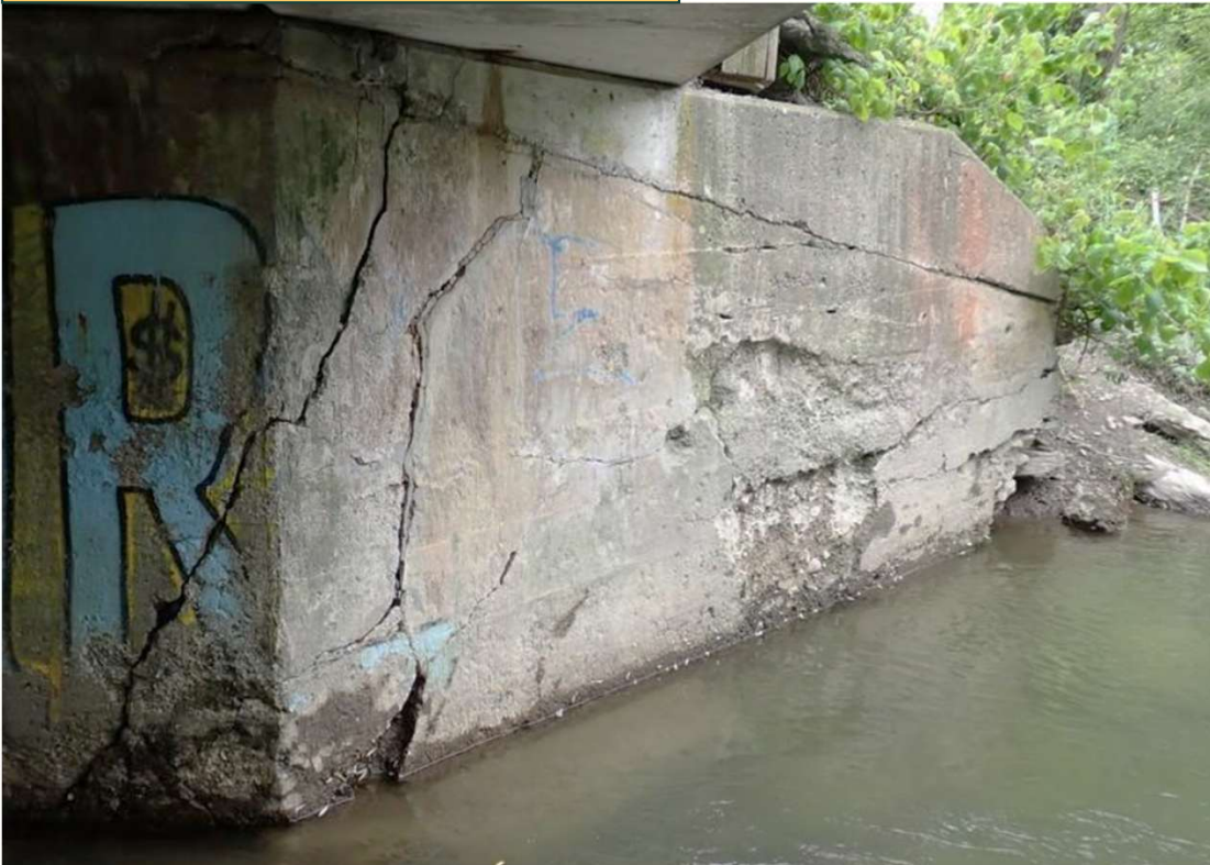
Cracks and Spalling of Concrete
