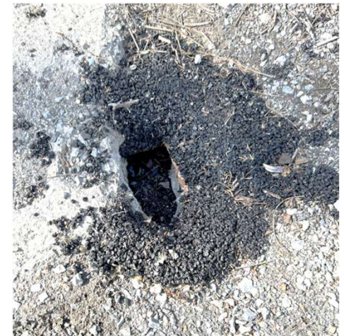
Holes in Box Beams Patched with Asphalt
